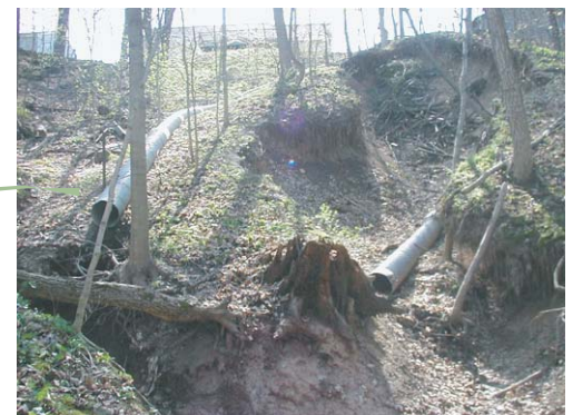
Gullies formed by storm drainage in nearby Ackerman Creek (pipes were probably added to control erosion, but will not solve the problem).
