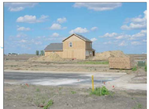
Extensive disturbed areas with no erosion control lends to massive sedimentation of Tenmile Creek.
