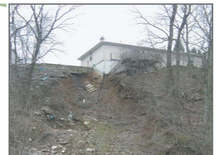
Development such as this in nearby Farm Creek Watershed can be problematic if erosion of slopes is not taken into account.
