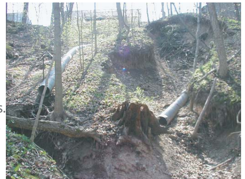
Westwood Park Tributary; gullies formed by storm drainage (pipes probably added to control erosion, but will not solve the problem).
