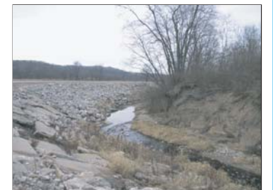
Stream channel erosion can lead to expensive infrastructure projects, such as the riprap placed along Veterans Drive (above) and the placement of a concrete channel bed to protect a sanitary sewer line (below).
