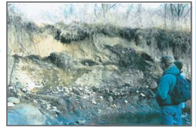
Streambank erosion along Ackerman Creek is a major source of sediment in the stream system (above).
