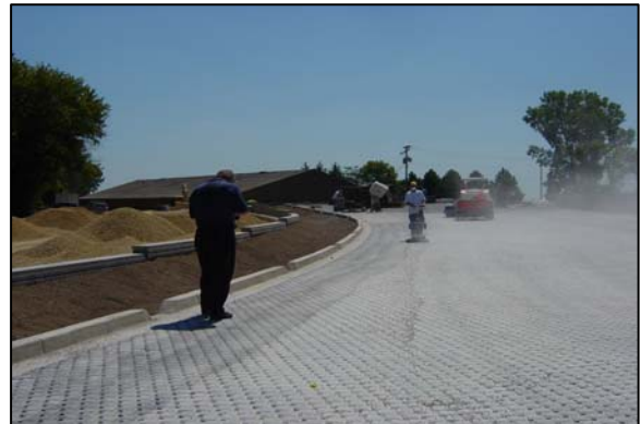
Fig. 8 Engineered grassed swales being constructed in the same parking lot. Notice the curb cuts that allow stormwater to enter the drainage system.
